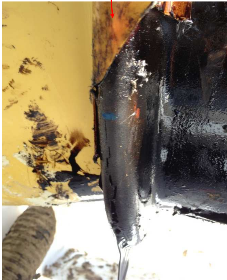
FIGURE 3 BUCKLING DEFORMATION AT 16TAN LEAK SITE
