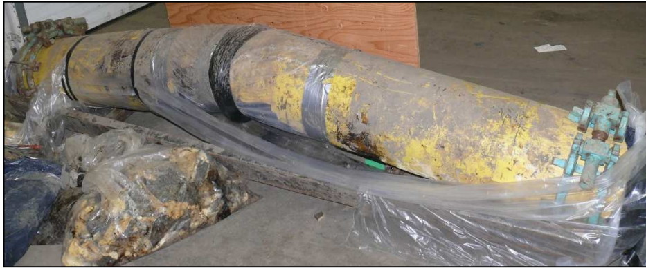
FIGURE 1 AS-RECEIVED PIPELINE FAILURE SAMPLE
