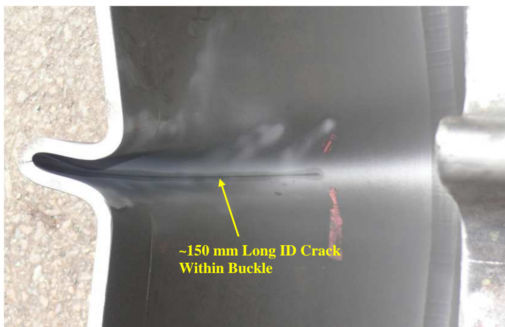
FIGURE 14 INTERNAL CRACKING WITHIN APEX OF THE ENDS OF THE BUCKLE ON EITHER SIDE OF FRACTURE ZONE
