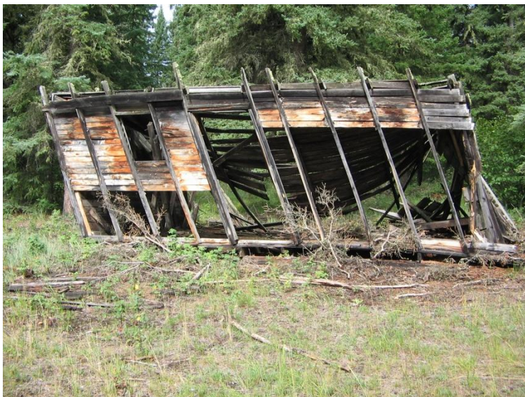
Figure 3-1 A dilapidated Heritage Site in Northern Saskatchewan
