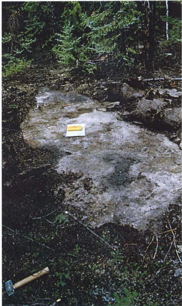
Johnson Lake Grey Granite exhibits widely spaced fractures. Outcrops clear of vegetation are uncommon in this stone.
