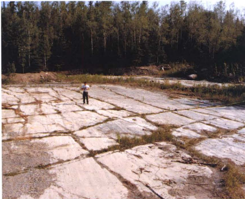
Fracture pattern in buff marble. Note vegetation indicates deep penetration of major fractures.
