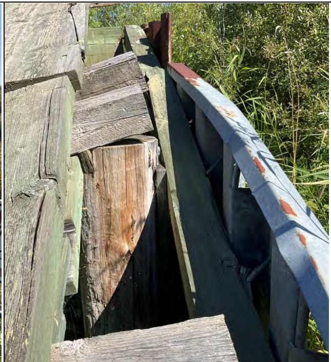
Image 2. Water retention structure (location #3 on Figure 3-2) with sheet piling and walkway damaged due to frost heaving.
