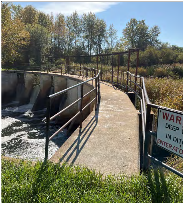
Image 1. Birch River Dam (structure #40 on Figure 3-2), the largest of the water control structures in the Cumberland Marsh system and approaching end of life.
