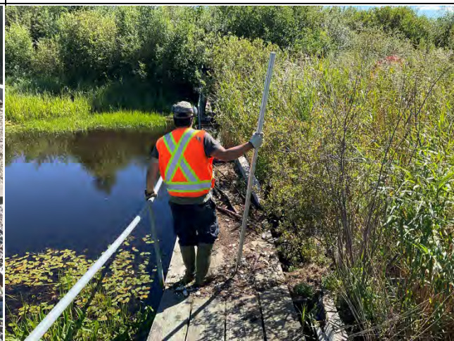
Image 4. Crest of the water control structure (Location #3 on Figure 3-2) showing damaged walkway and overgrown vegetation.
