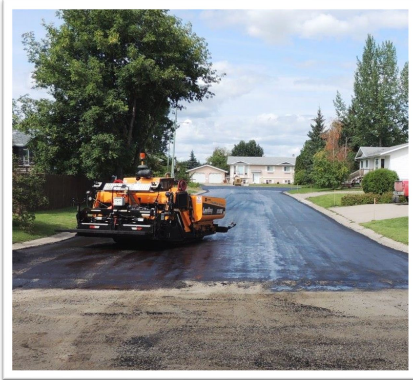
Palenchuk Place rehabilitation work in progress (Photo courtesy: City of Meadow Lake)
