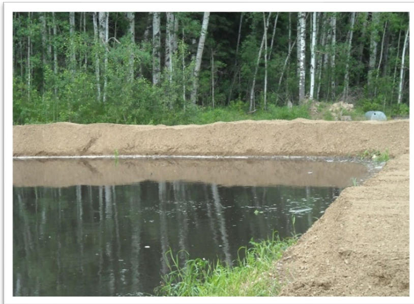
Reinforced berm around East Trout Lake (Photo Courtesy: Northern Saskatchewan Administrative District)
