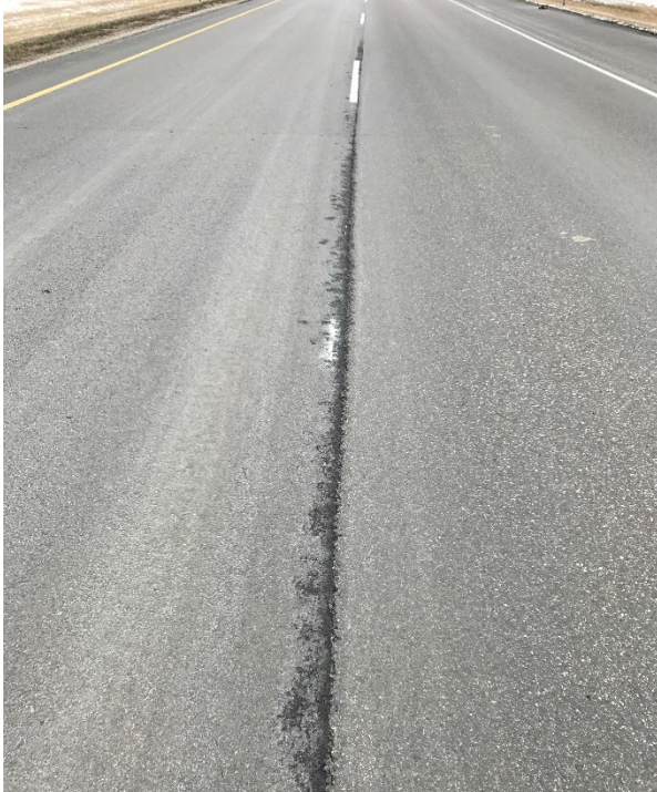
Figure 19: Improper Matching of Longitudinal Joint
