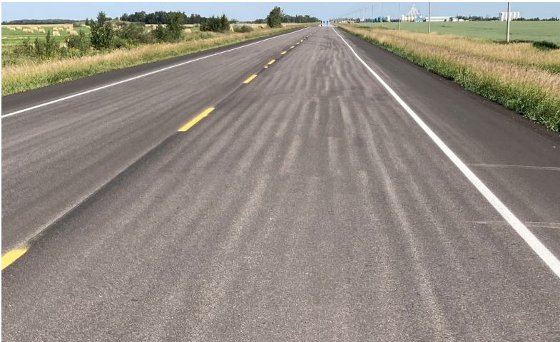
Figure 26: Roller Marks, Asphalt Film Loss
