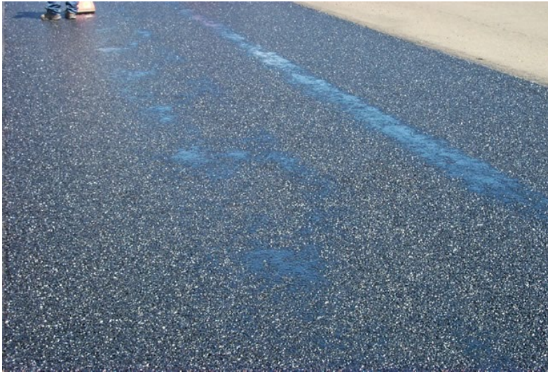
Figure 15: Excess Asphalt Binder
