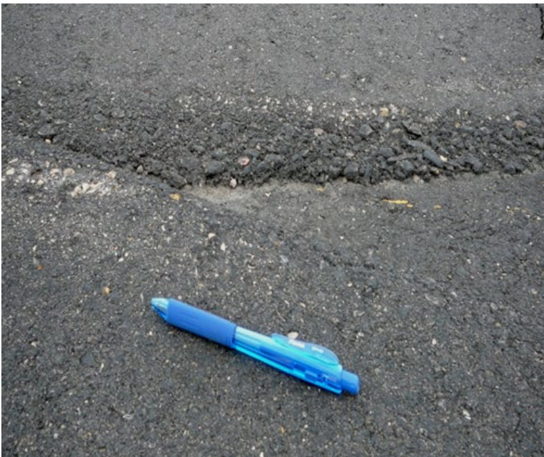
Figure 20: Improper Matching of Longitudinal Joint
