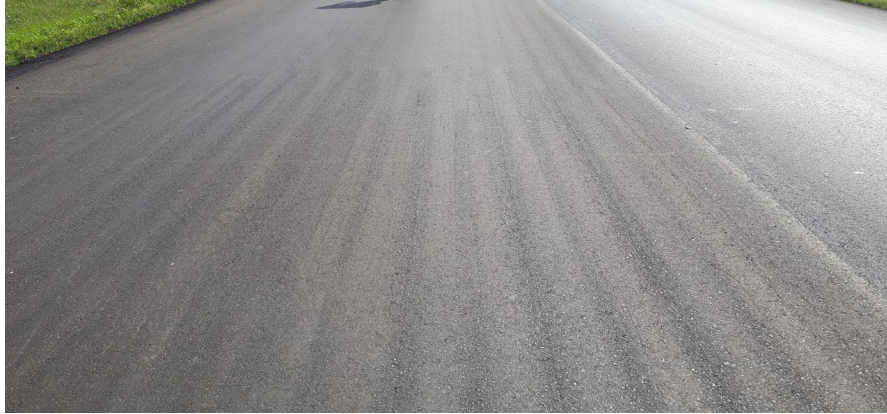
Figure 27: Roller Marks, Ridges and Depressions
