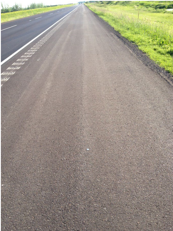
Figure 16: Insufficient Asphalt Binder
