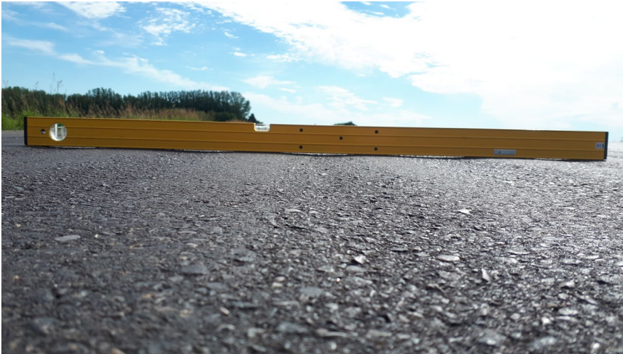
Figure 28: Roller Marks, Ridges and Depressions
