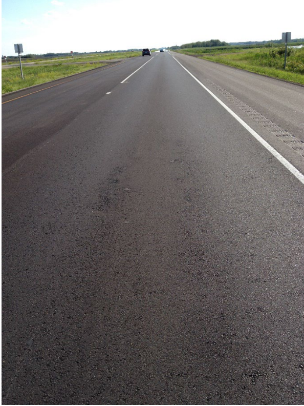
Figure 10: Moderate and Severe Segregation
