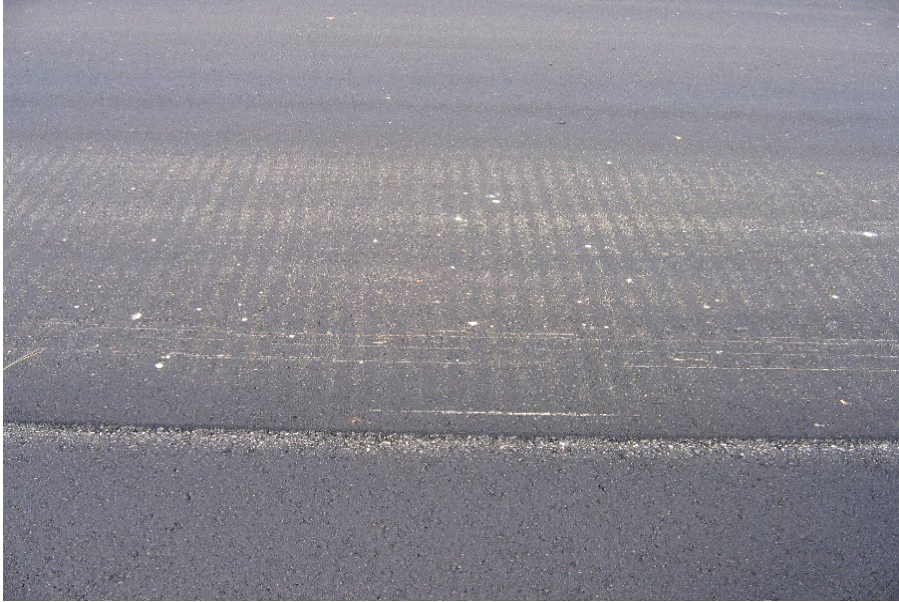
Figure 29: Roller Marks From Vibrating Steel Drum
